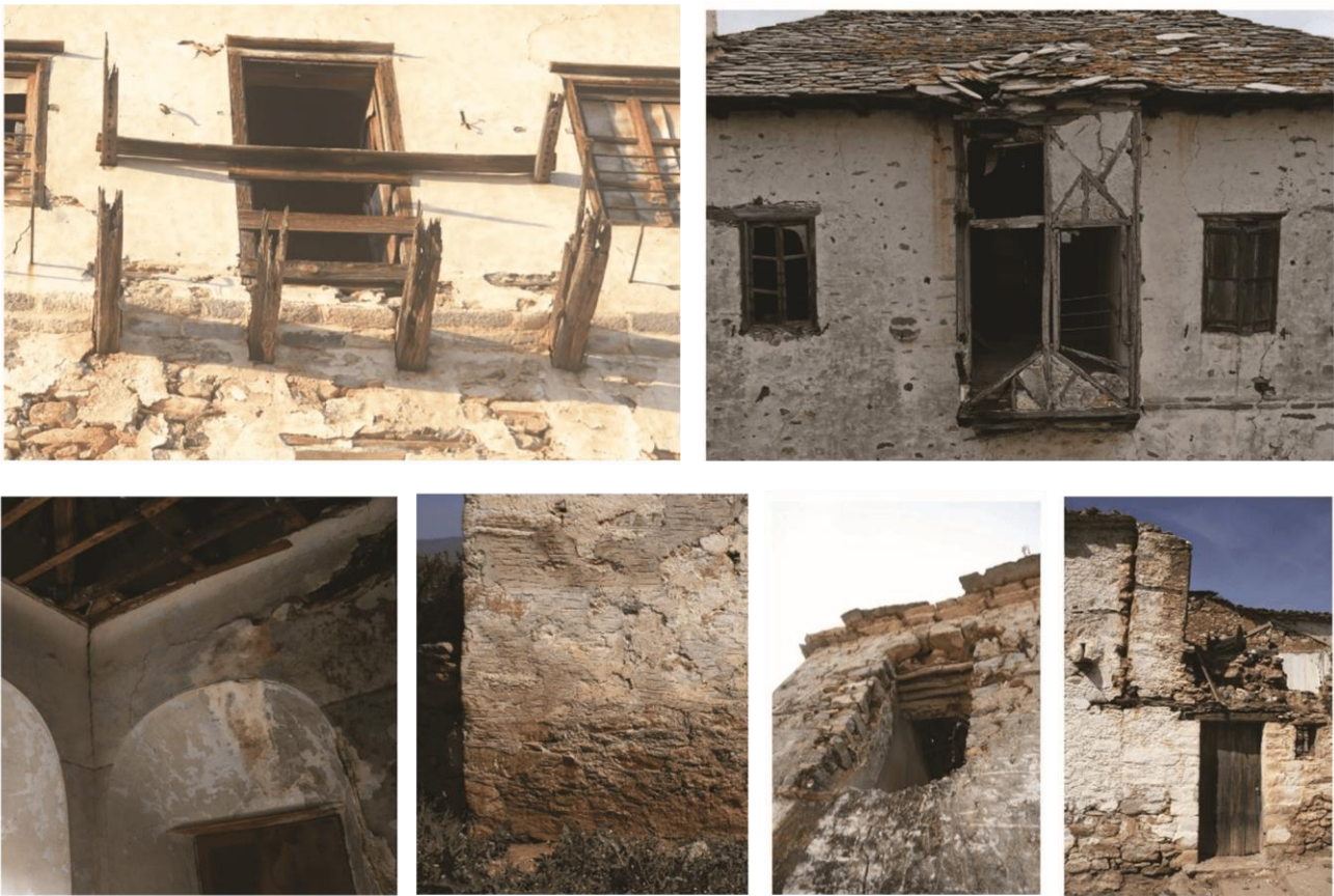
Fig. 7: Examples of structural problems of the complex
